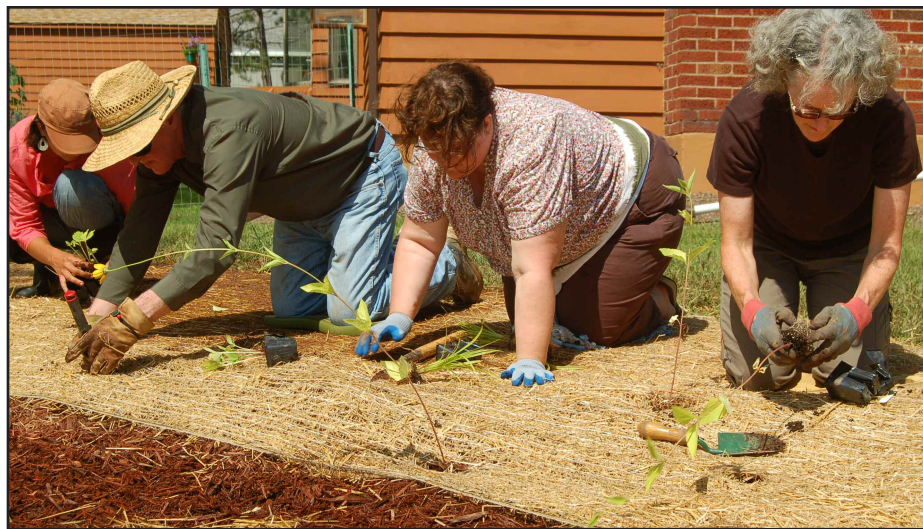
Rain garden planting in Duluth, Minnesota. Photo by Chris J. Benson.
